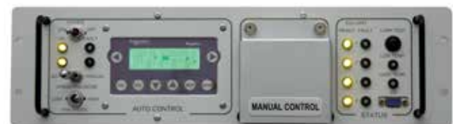
Central Control System
